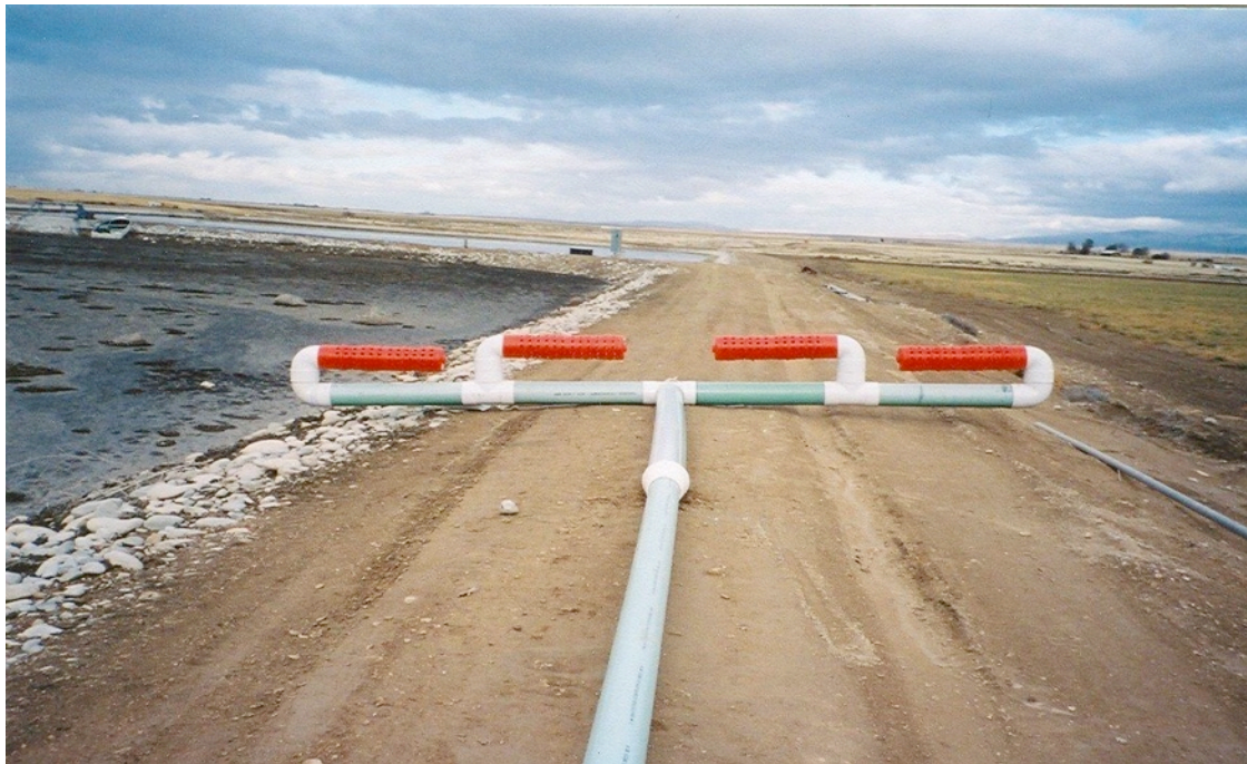
Example of a similar suction piping manifold showing height of the risers off the bottom of the lake (photo courtesy Seven Star Enterprises, LLC, Mankato, MN)
