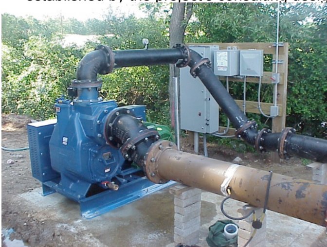
Gorman Rupp V6A60B self-priming pump is lifting water 15' from the lake and pumping it through the six-inch Model VA-1200 Venturi Aerator which is submerged in the lake
