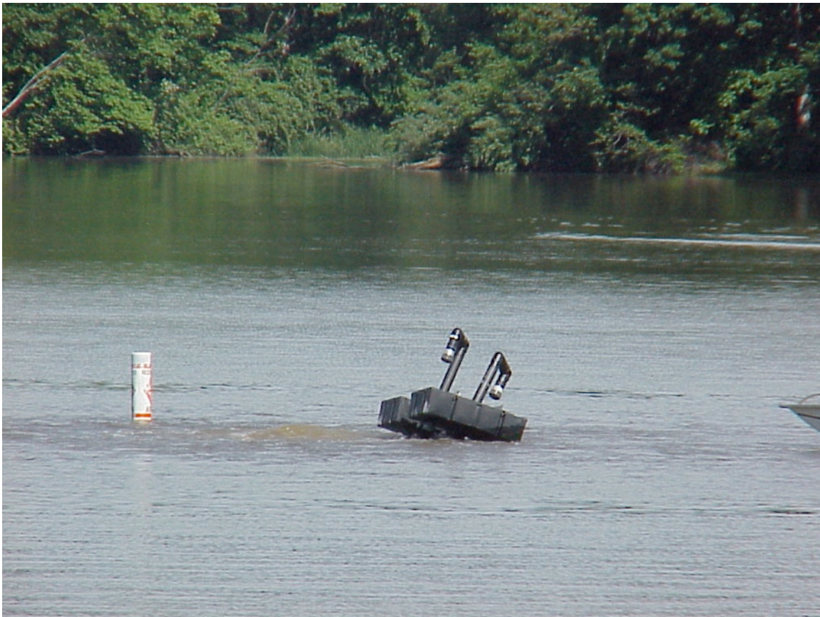
Breakthrough at the surface is very visible as is the eddy that is created allowing additional oxygen transfer at the air/liquid interface of the lake. The two air intake hoses for the venturi aerator are located
